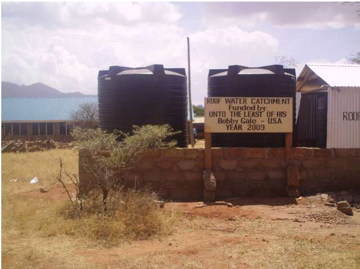
Installation of water tanks for roof catchment at Wamba Secondary School in Northern Kenya
