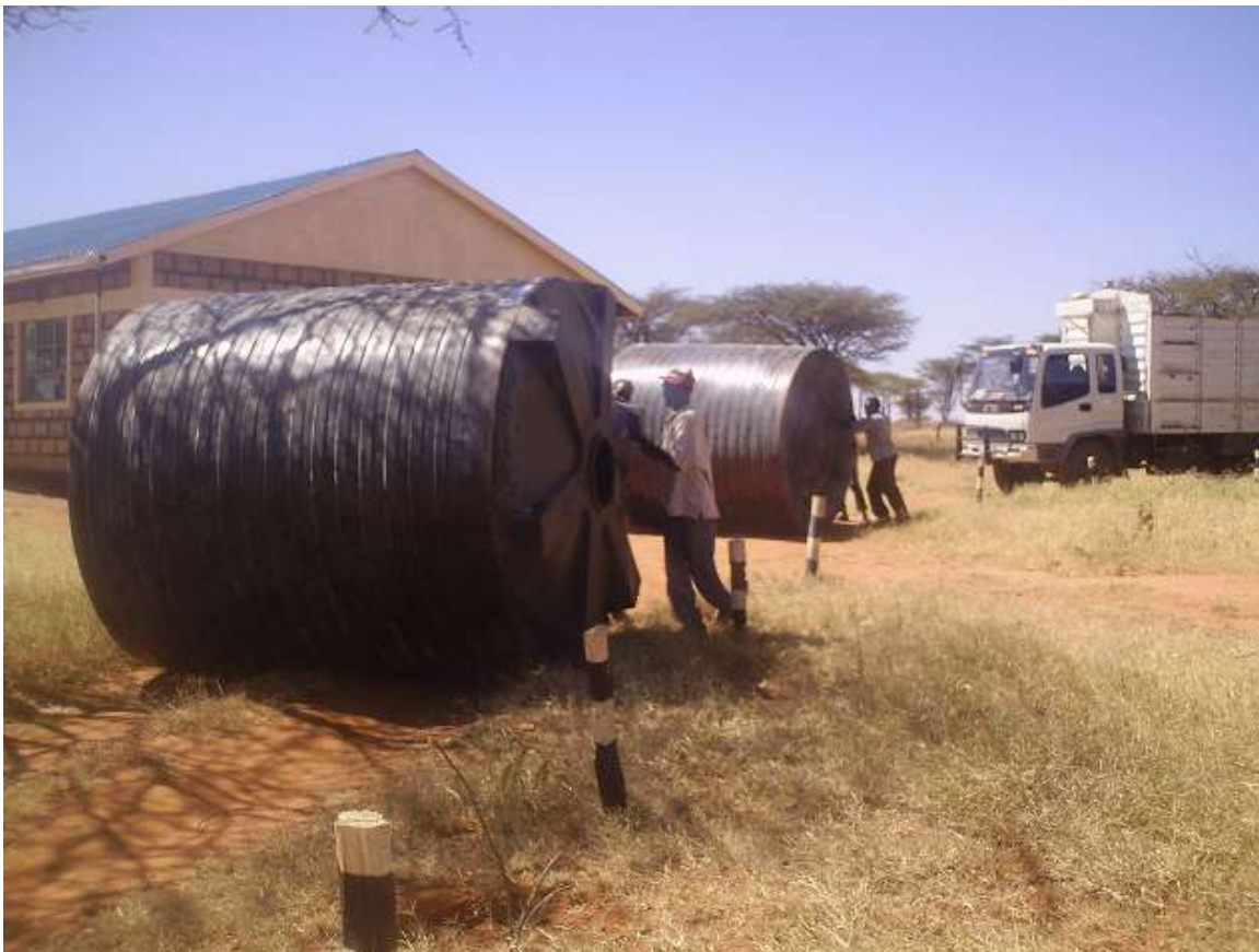
Rolling of tanks to site of installation in Wamba secondary school Northern Kenya. Thanks to Unto the Least of His – Bobby Gale USA.
